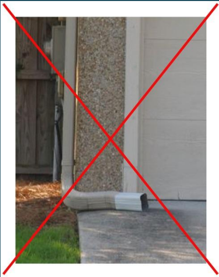
Downspout over impermeable surface
